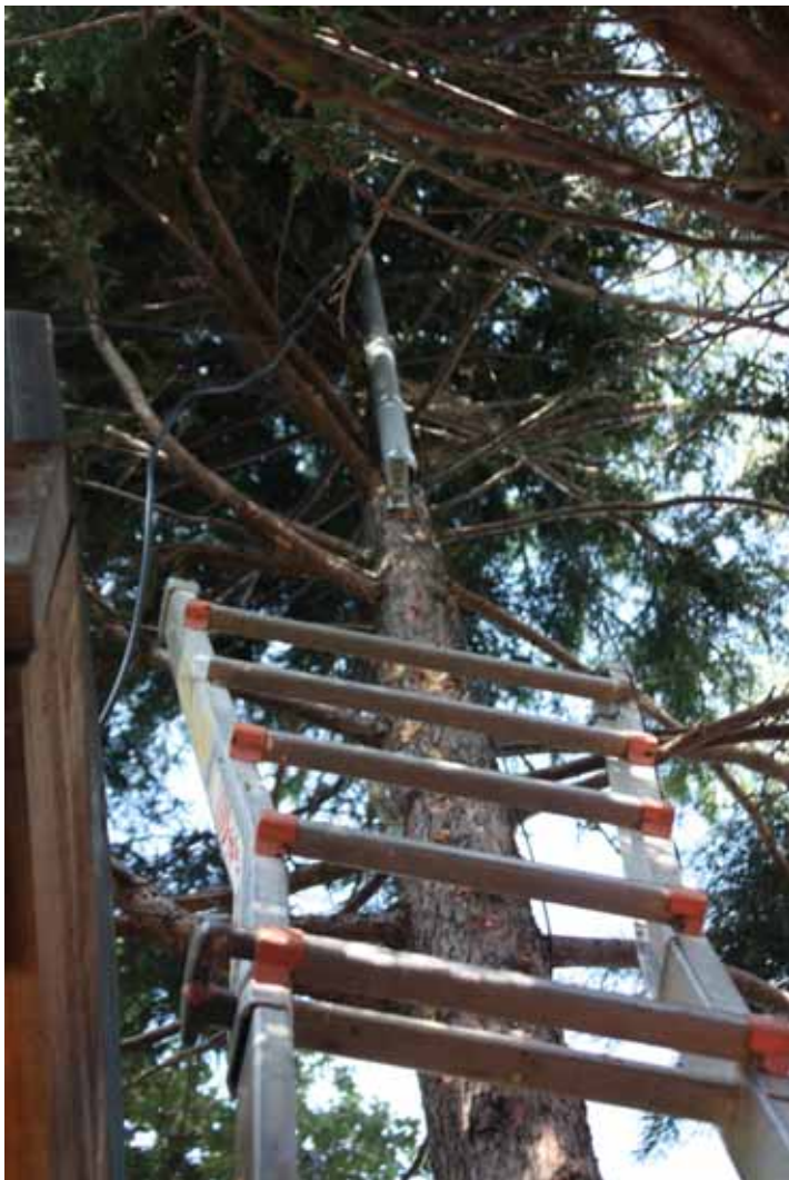
Pole mounted more than half way up the tree by Trevor ↑
